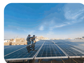
Rooftop PV array Illustrative photo
